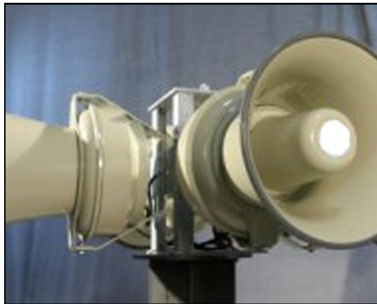
A typical high audio siren installation.
